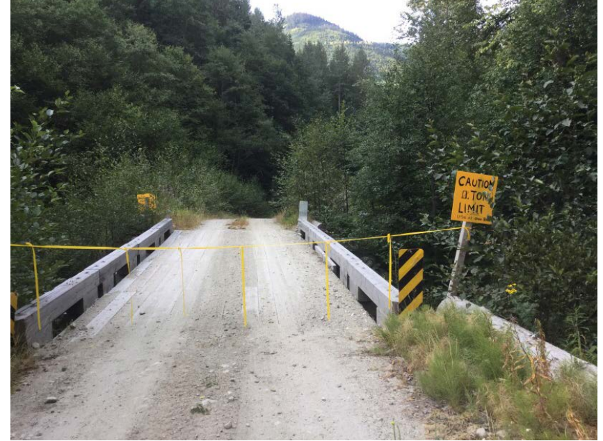
Updated load rating sign and notification at right approach
