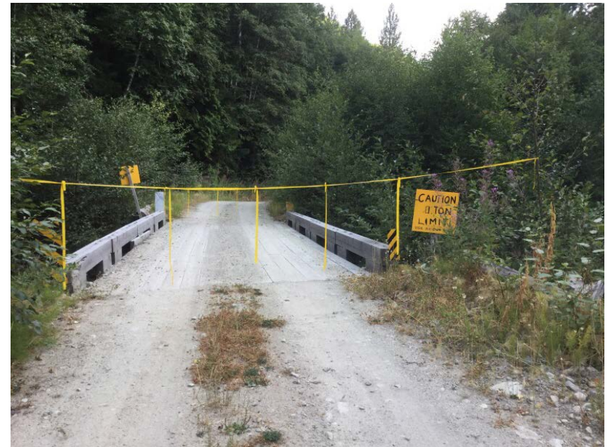
Updated load rating sign and notification at left approach
