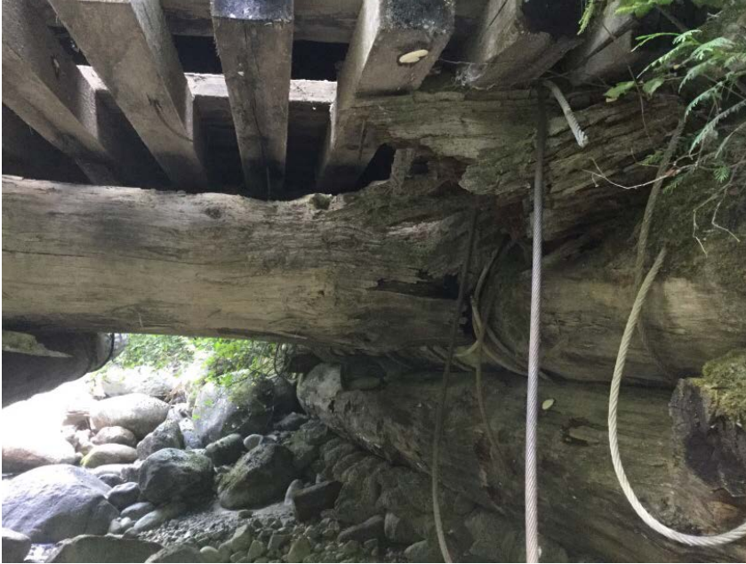
Stringer condition at left bank
