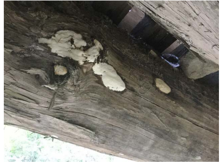
Log stringers under steel girder in poor condition
