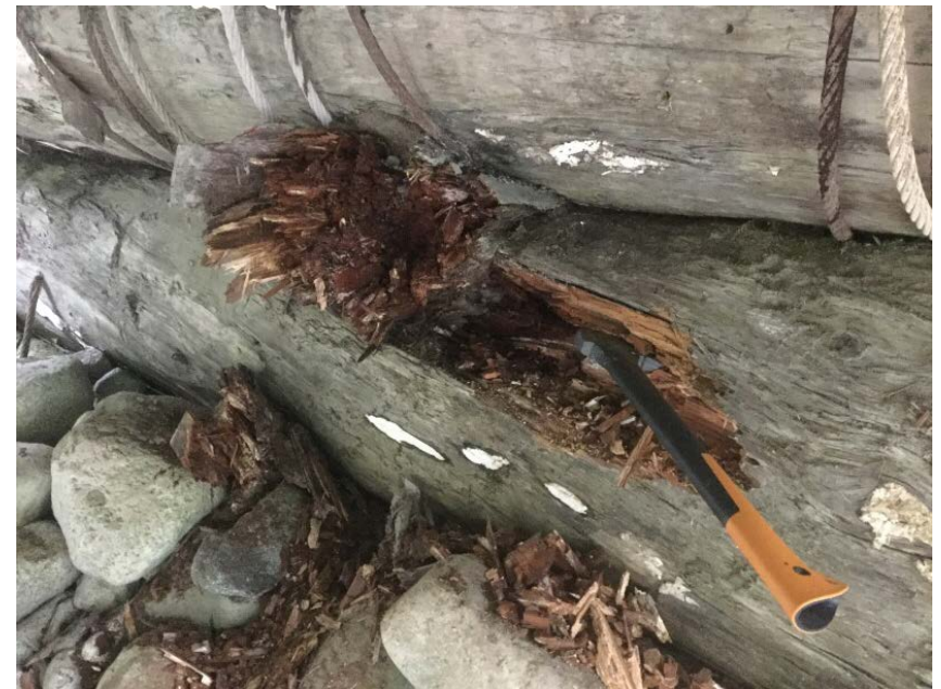
Log crib supporting stringers in poor condition
